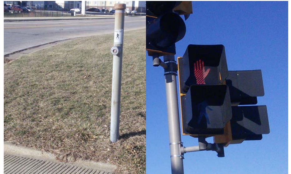
With a small pushbutton that lacks a tactile arrow, vibrotactile indicator, locator tone, and most other accessibility features, this pedestrian signal scores 40 on the combined compliance index.
