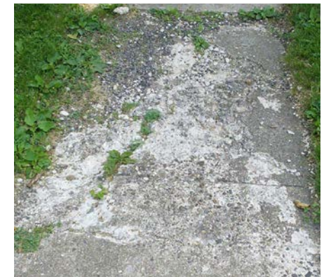
Surface Condition: Spalling
