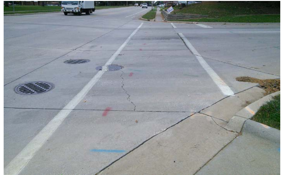
With a width of 92 inches and a cross slope of 6.3 percent, this crosswalk at a stop-controlled intersection scores 70 on the combined compliance index.
