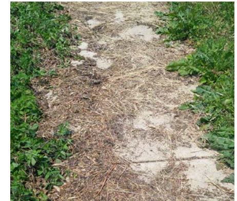
Surface Condition: Dirt
