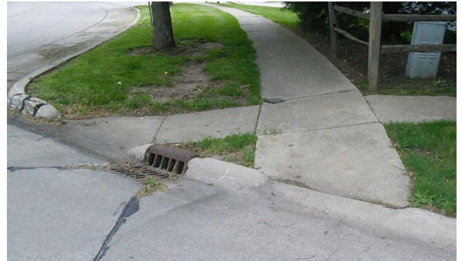
With multiple accessibility issues, this ramp scores 31 on the combined compliance index. The ramp lacks a detectable warning surface, the left approach is obstructed by a water valve, and many of the cross slopes are 10 percent or above.
