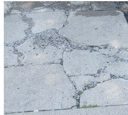
Surface Condition: Cracking
