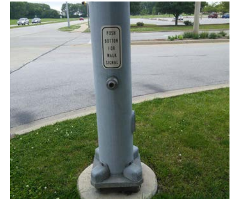
Traffic Signal Pole
