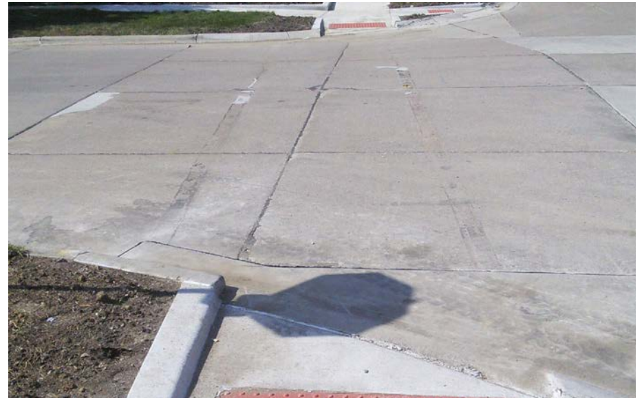
In this crosswalk, the standard painted markings and the stop bar are worn, almost to the point of being unrecognizable.
