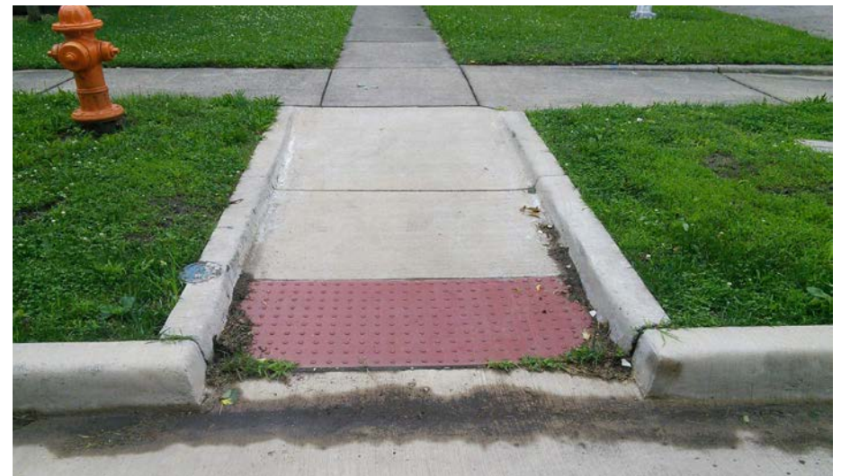
With a width of 60 inches, a minimum landing dimension of 48 inches, truncated domes that fill the width of the ramp, and all slopes within the compliant ranges, this ramp scores 100 on the combined compliance index.
