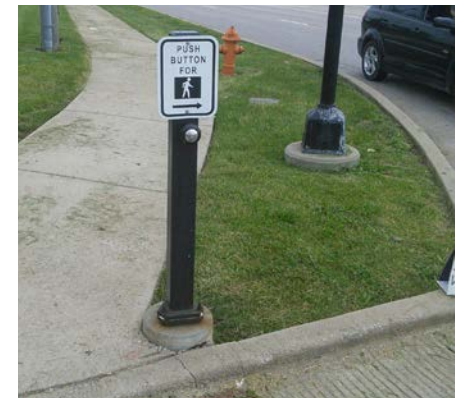
Pushbuttons within 10 Feet of the Curb
